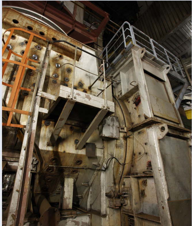
Coal bunker and coal mill
