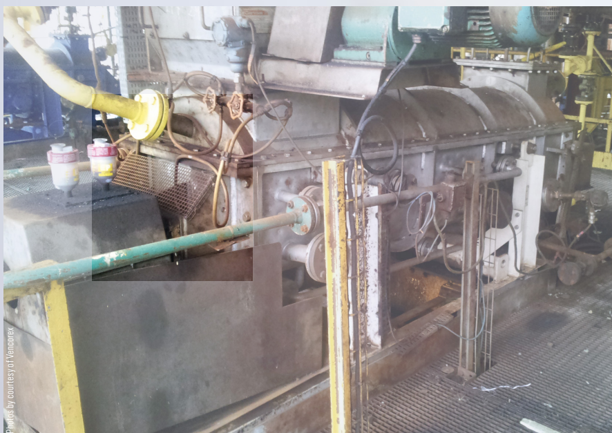
Paddle dryer in operation for the production of TDI
